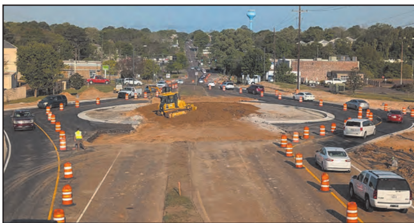
University Avenue roundabouts being constructed in Oxford, Mississippi. Photograph by Matt Nichols, April 14, 2025.
